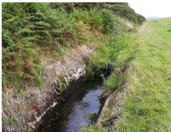
Plate 3-13 Headrace toe drain (TD1) showing concrete-lined channel (May 2025)
